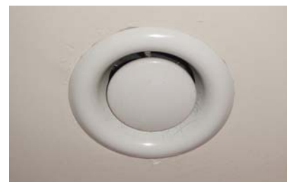
Ceiling air supply vent. Source: MosArt Architecture.
